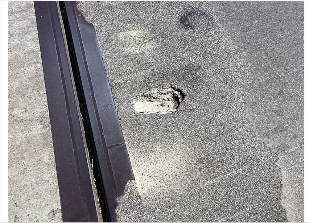
A approach pavement pothole
