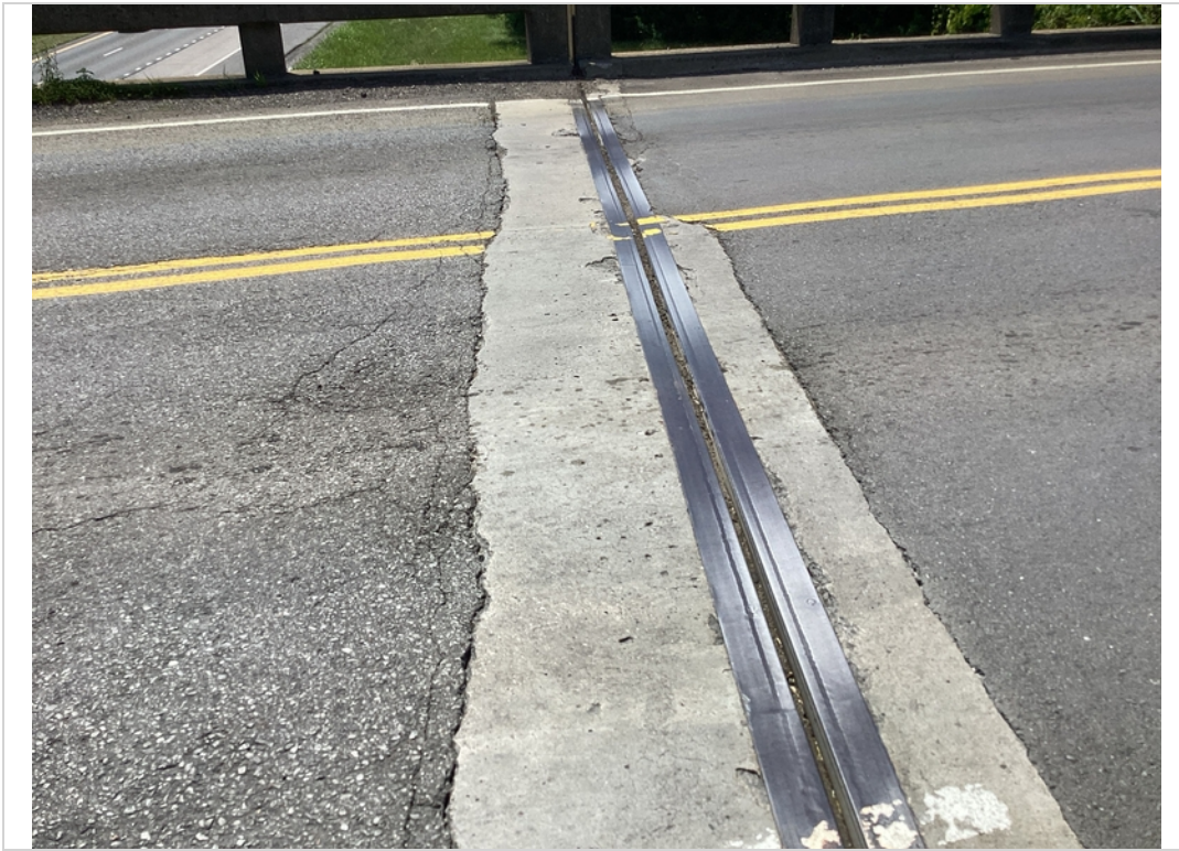
B approach wearing surface area of map cracking full length
