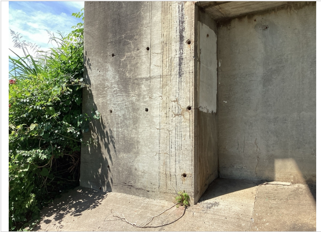
Abutment 2 cap map cracking
