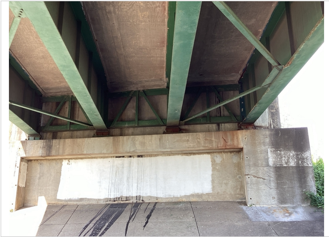
Abutment 2 bearings B - D moderate corrosion
