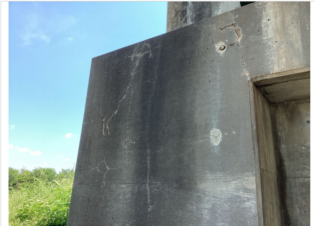
Abutment 1 cap random hairline cracks w/EFF. throughout
