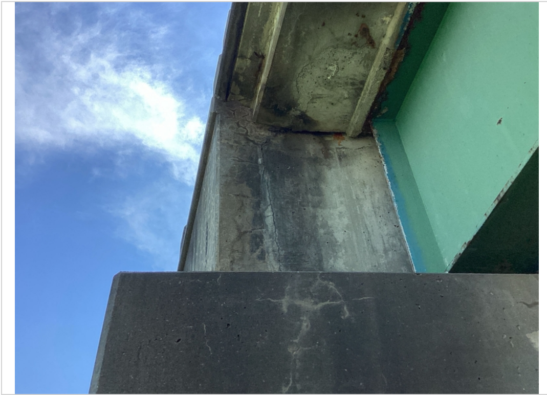
Abutment 1 backwall Rt. Side 1/16" vertical crack
