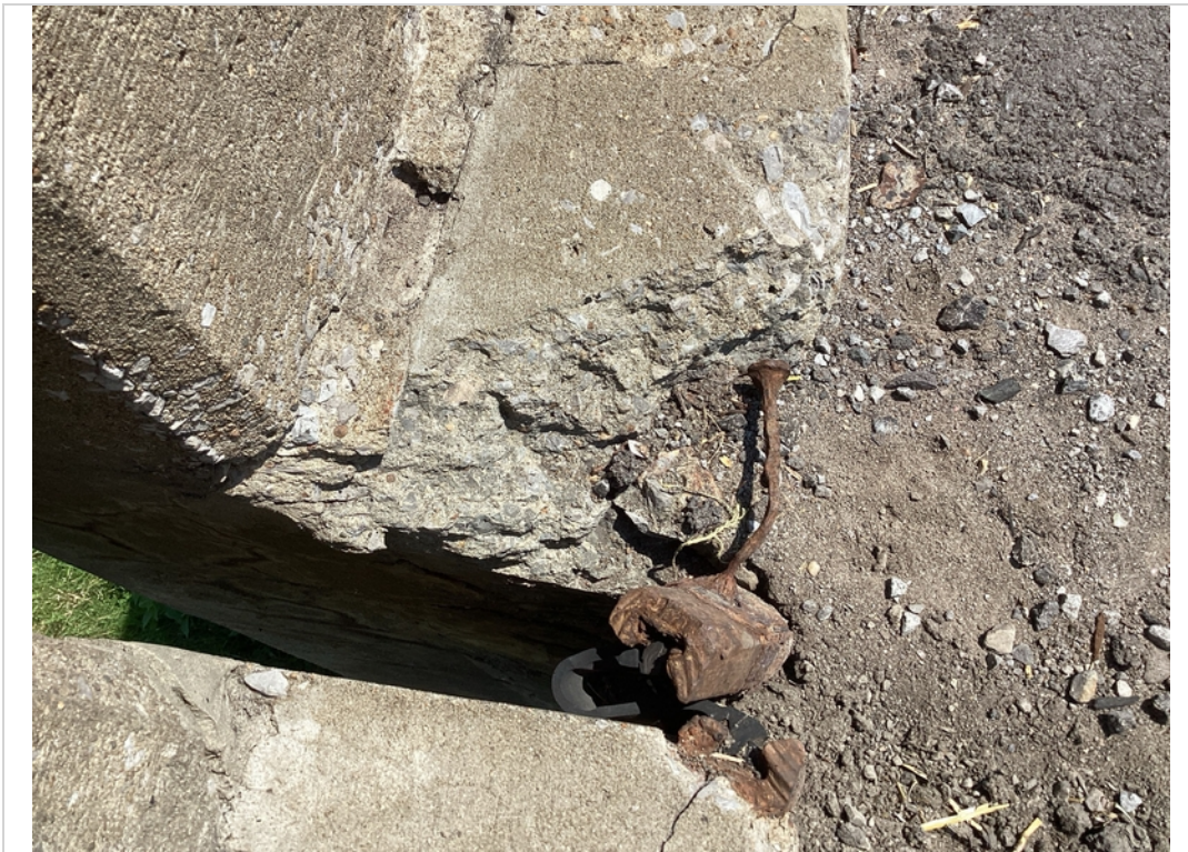
Bridge parapet right side near A approach joint spall with exposed steel
