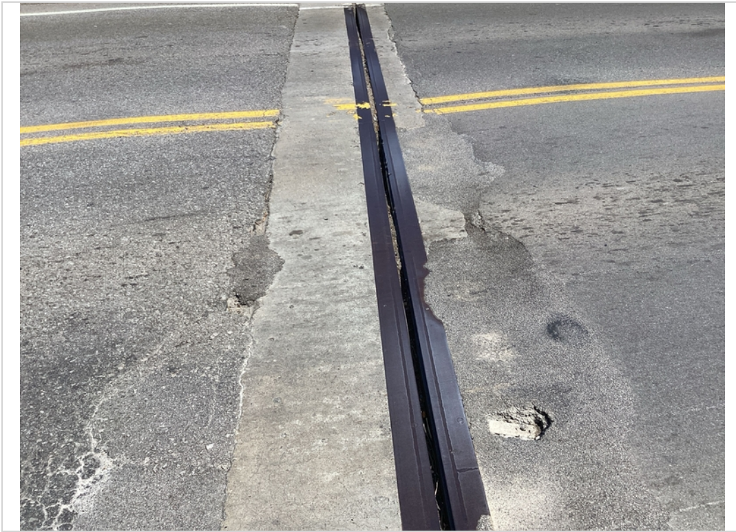
A approach joint filled with light debris
