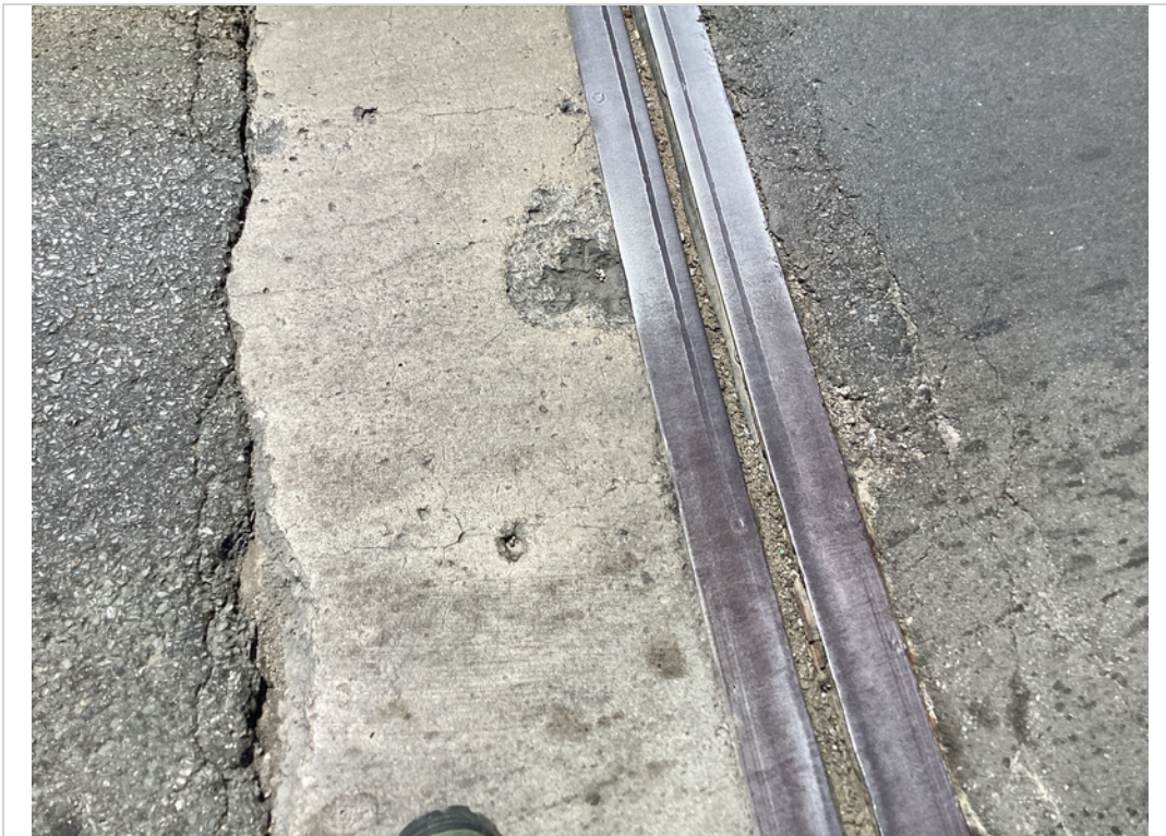
B approach wearing surface left side pothole
