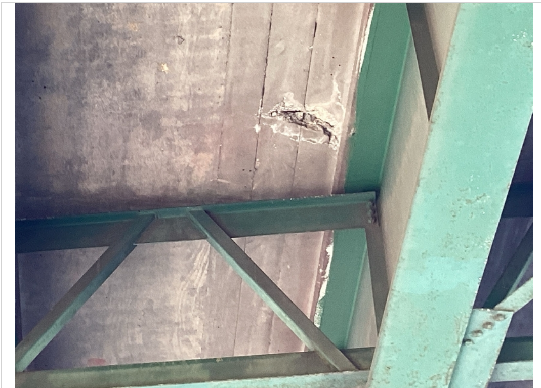
Spall in Bot Deck Bay 2 Span 1
