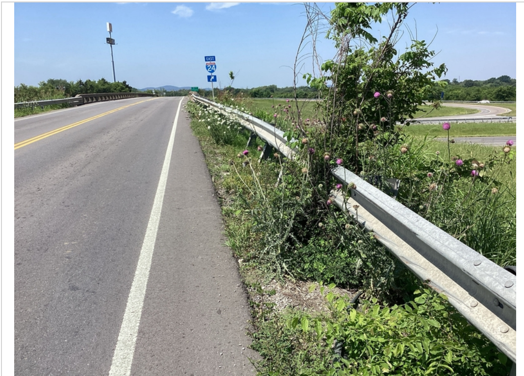
A approach Rt. side guardrail damage
