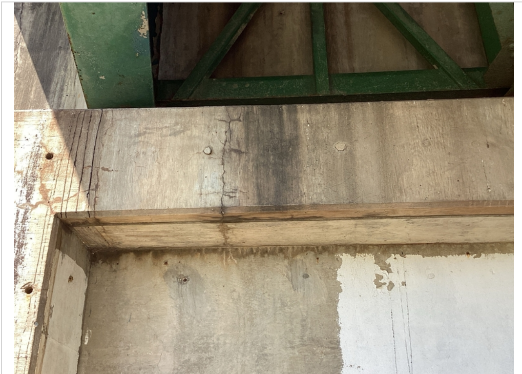
Abutment 2 cap 1/16" vertical cracks throughout
