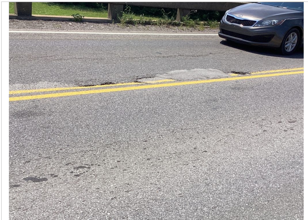
Span 2 near B approach area of small potholes over A/C patches
