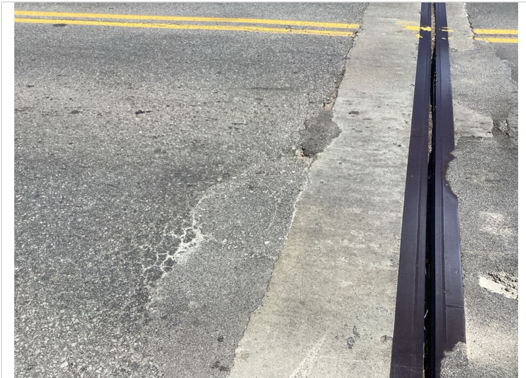
A approach wearing surface A/C patches
