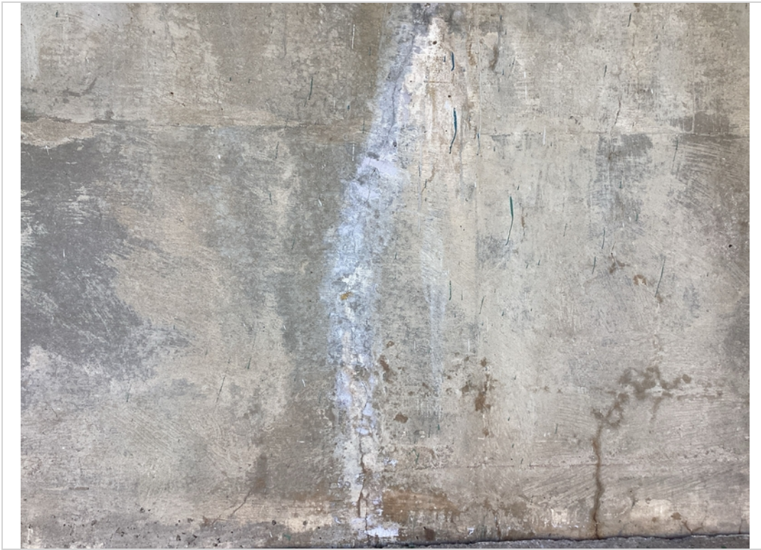
Abutment 1 breastwall Random hairline cracks w/EFF. Throughout
