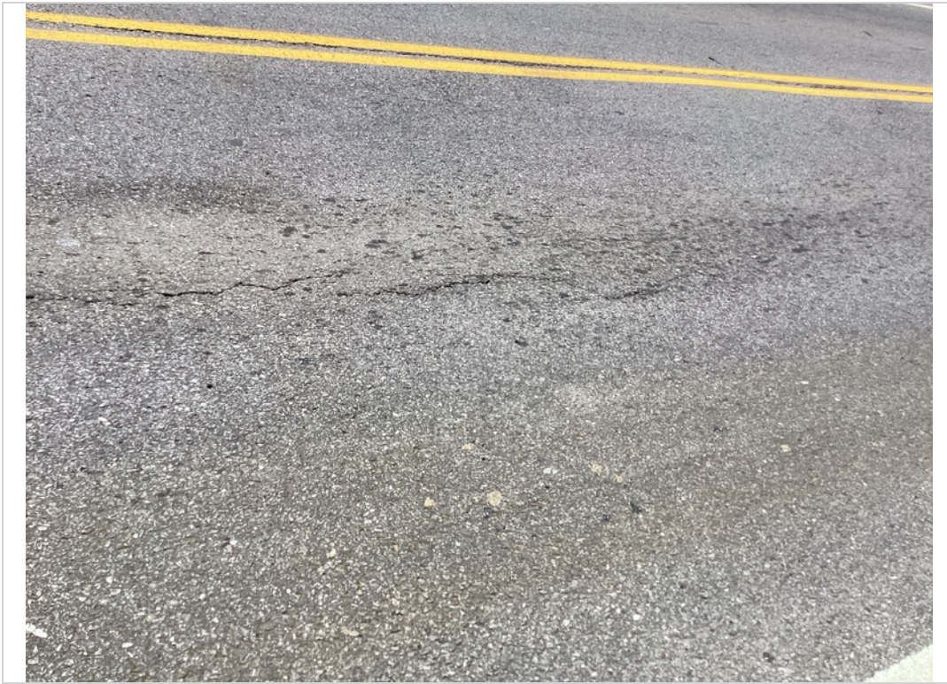
Span 1 near A approach 1/8" open longitudinal crack
