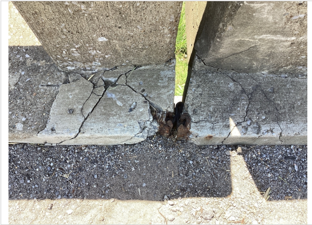
Bridge parapet left side near A approach joint area of delamination
