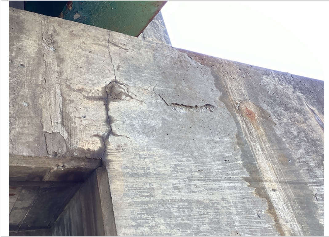
Abutment 1 cap Lt. side area of delamination
