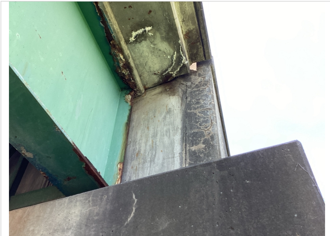
Abutment 2 Rt. Side backwall map cracking w/EFF
