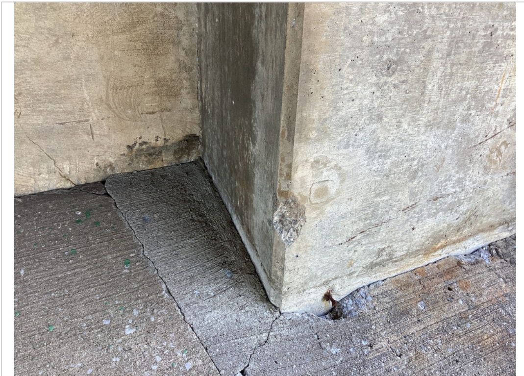
Abutment 1 cap Lt. side spall
