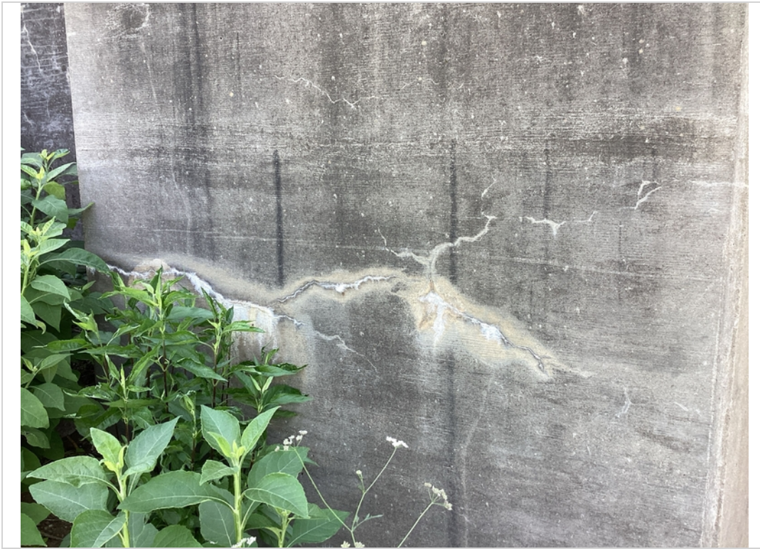
Abutment 1 Rt. Wing map cracks w/EFF.
