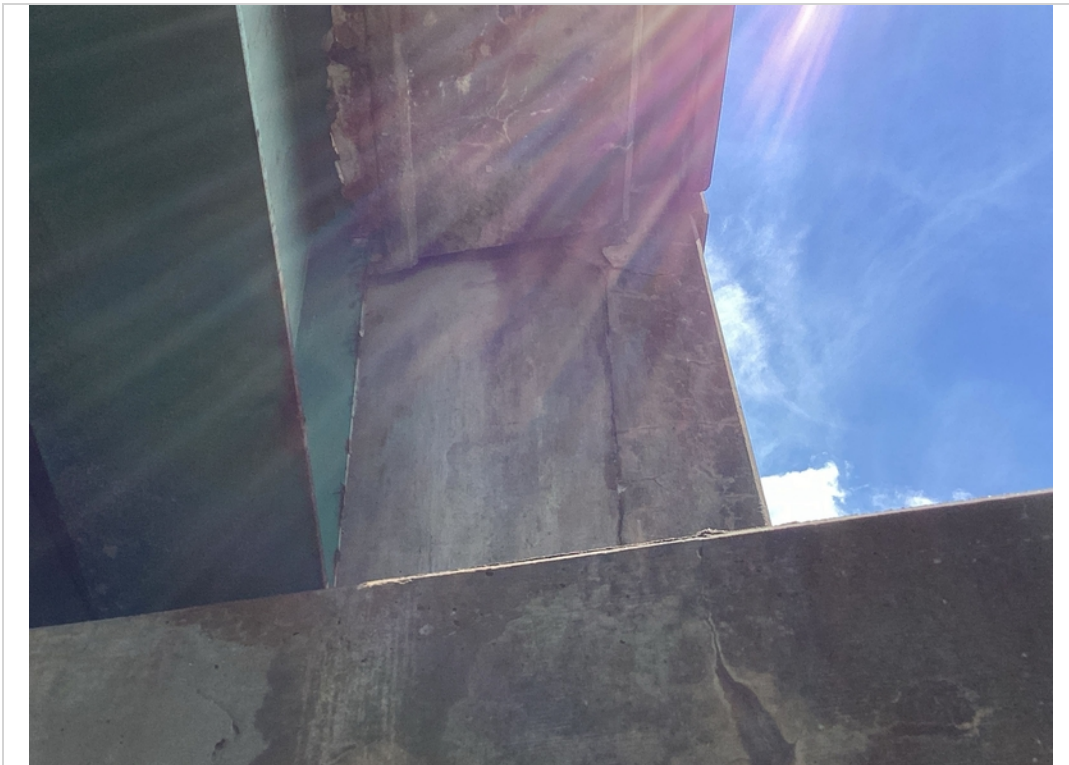
Abutment 1 backwall Lt. side 1/16" vertical crack
