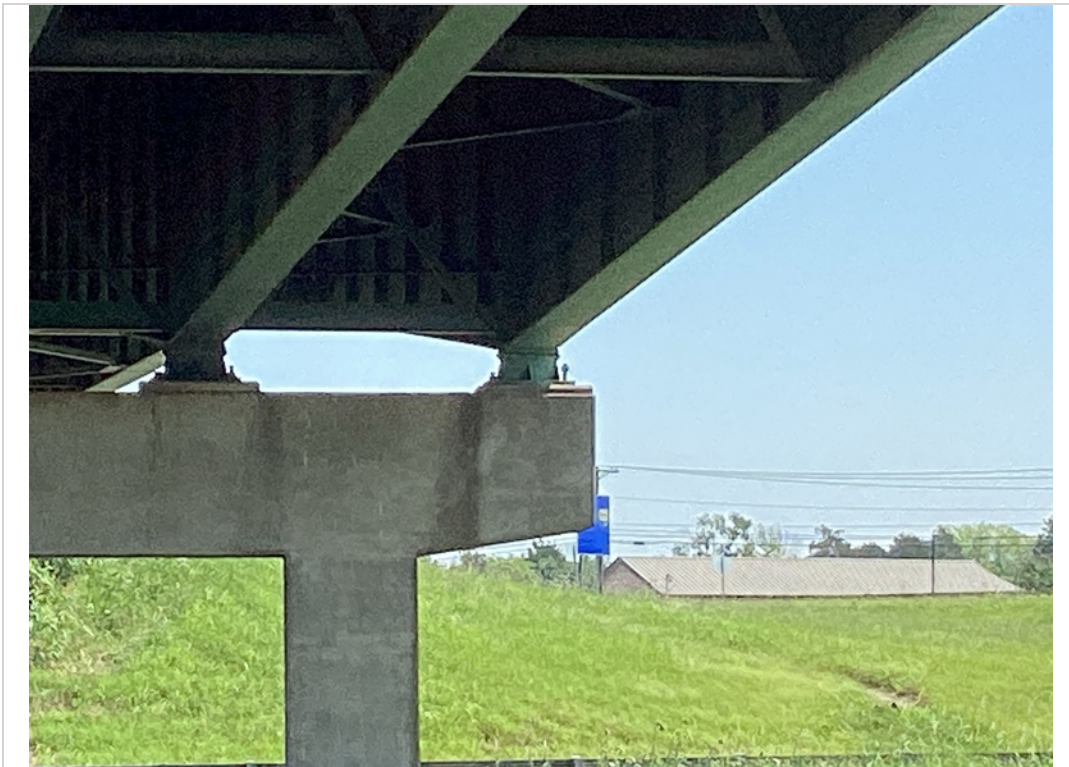
Bent 1 Lt. side loose nut at bearing A
