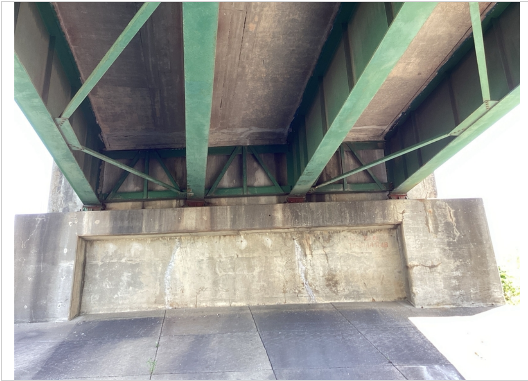
Abutment 1 moderate corrosion on bearings
