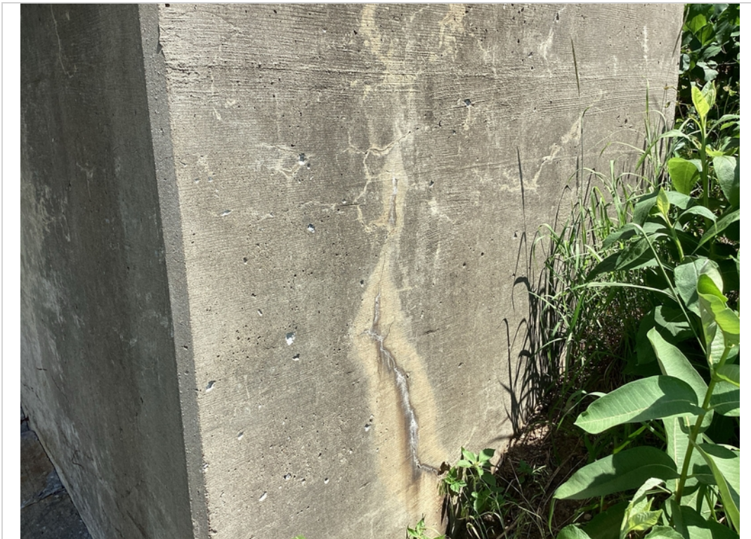
Abutment 1 Lt. wing map cracks w/EFF.
