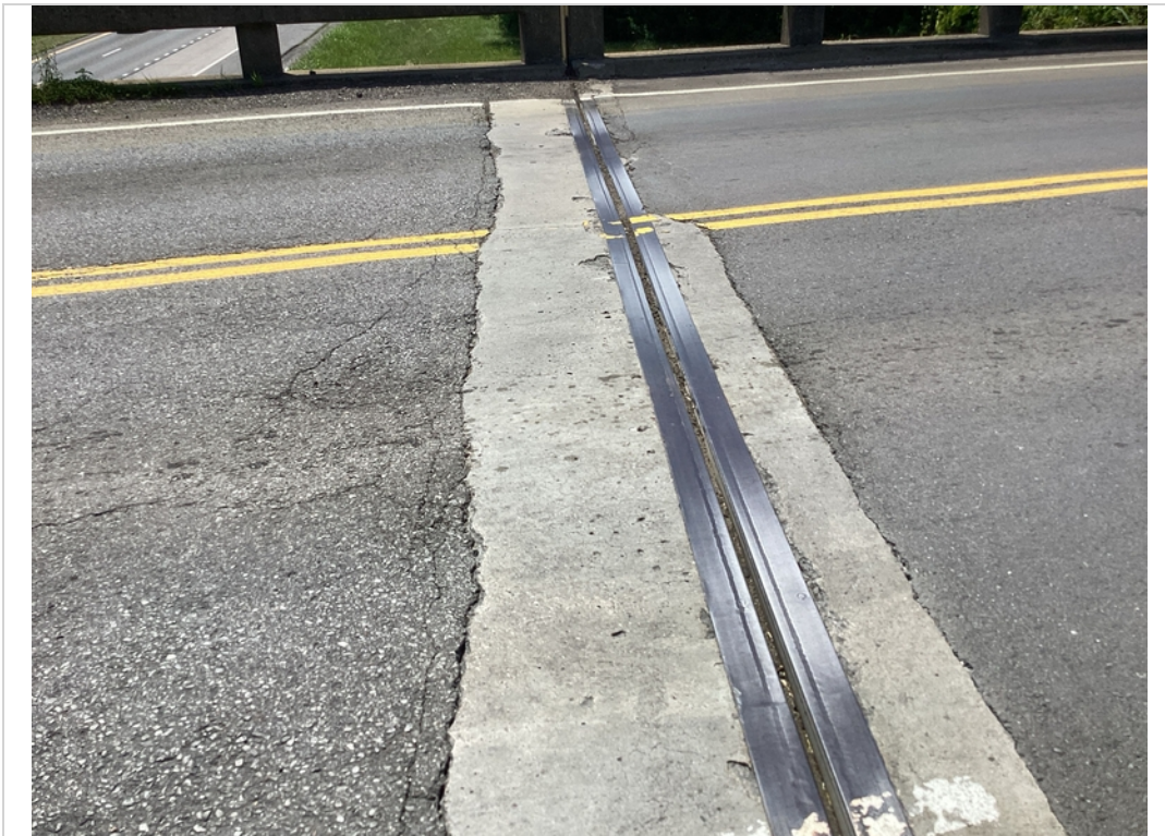
B approach joint filled with light debris
