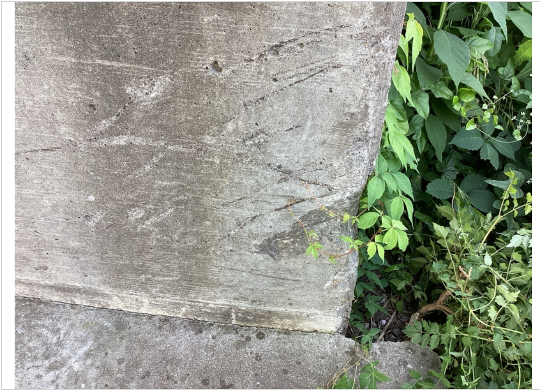
Abutment 2 cap Rt. Side spall
