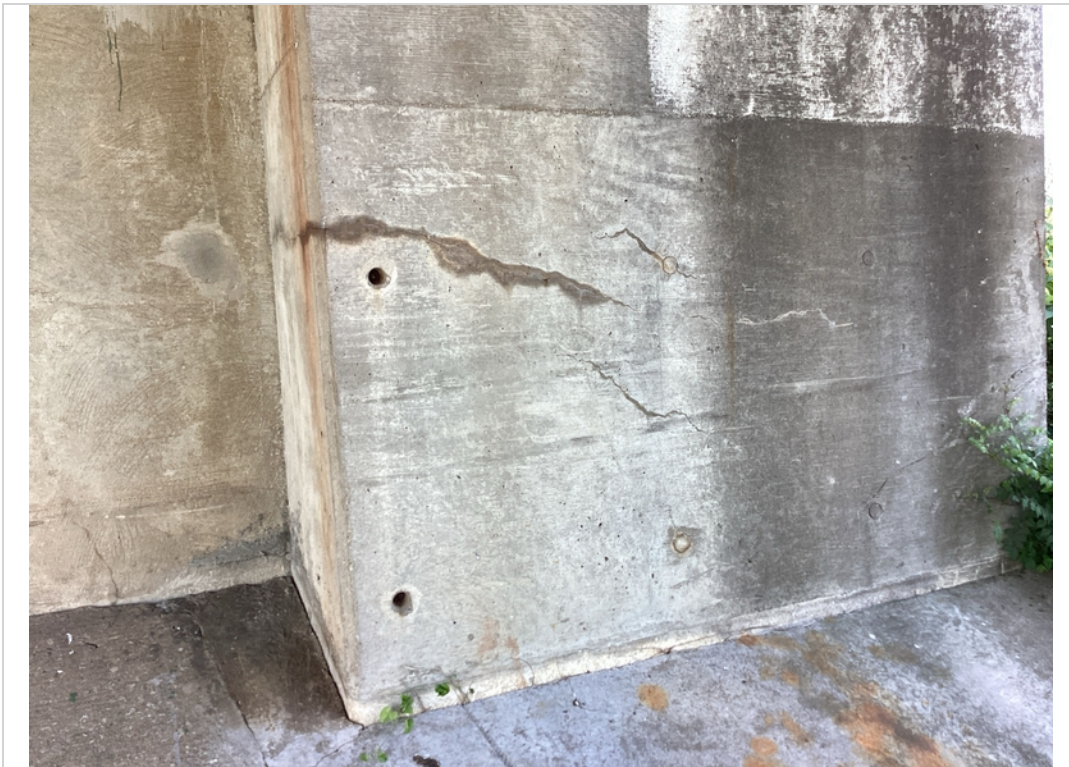
Abutment 2 cap random hairline cracks throughout
