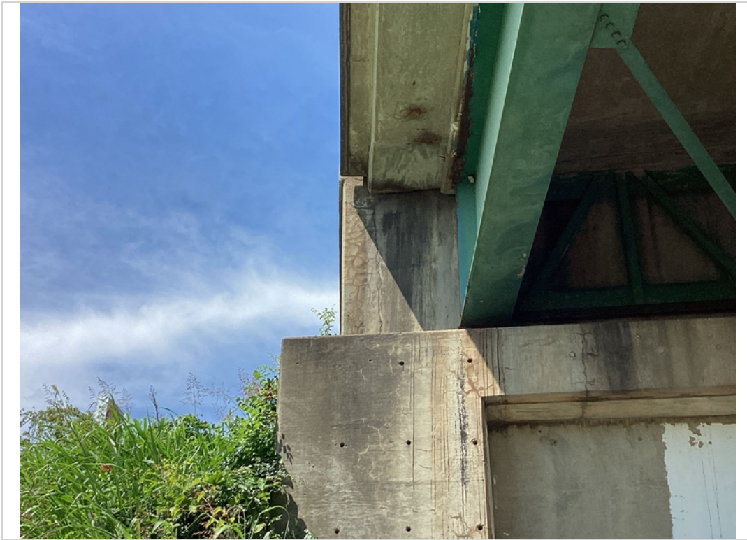
Abutment 2 backwall Lt. side 1/16" vertical crack
