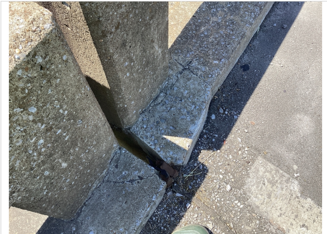
Bridge parapet right side near B approach joint area of delamination
